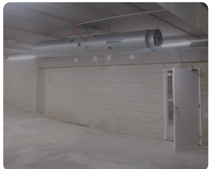
Jet fan AUO 290 in underground car park
