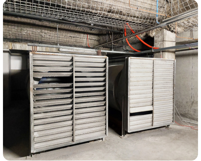
Pre-installation: Two worn-out fans reflecting years of heavy use
