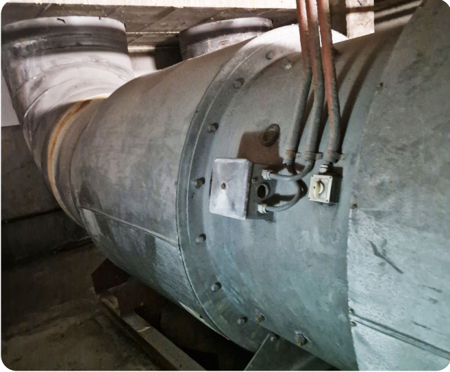
Space- and energy-consuming fan from the outdated system
