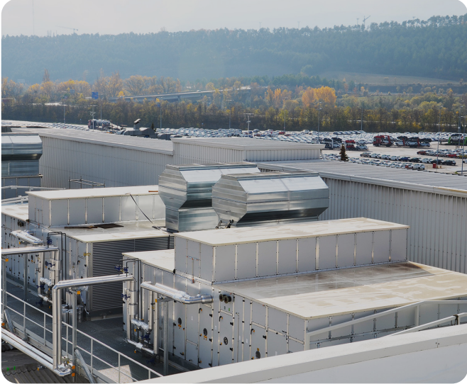
Energy savings, reduced weight and low noise were key factors in the upgrade
