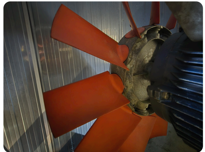
Worn-out fans – inefficient and outdated
