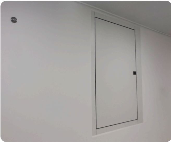
Smoke extraction damper installed in the corridor – ensuring safe and efficient smoke control during emergencies
