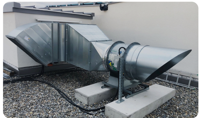
New bypass-solution with NOVENCO NovAx fan installed on the rooftop for optimal airflow and performance
