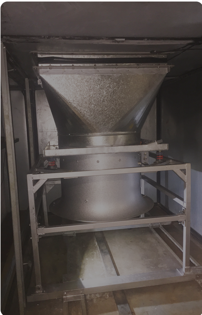
After retrofit- NOVENCO ZerAx axial fan
