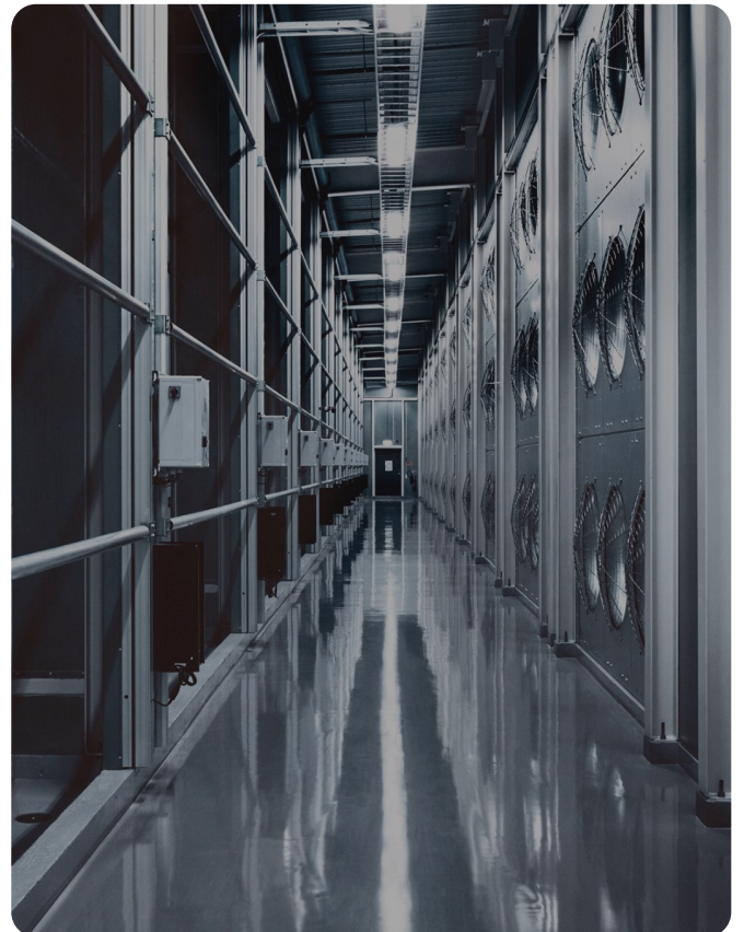
Inside one of the world's most energy-efficient data centers
