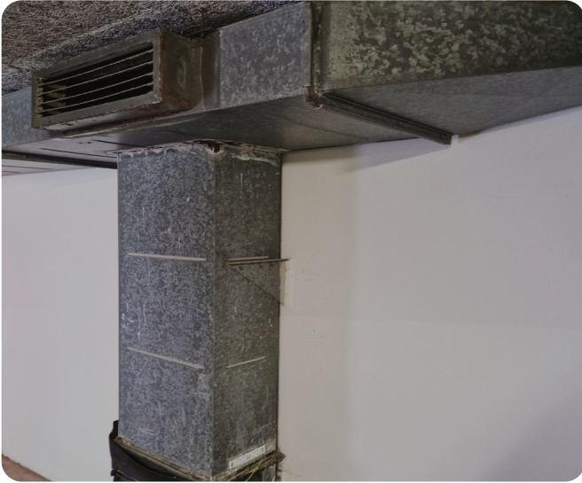
Before: outdated duct system – costly and inefficient
