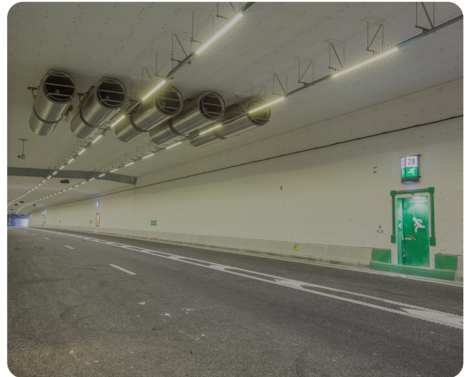
Jet fans handle both daily ventilation and emergency smoke control
