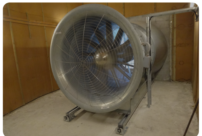
Newly installed ZerAx fan – compact design, maximum airflow
