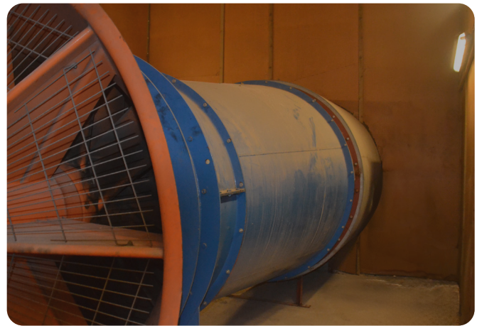
Old fan installation in the power house
