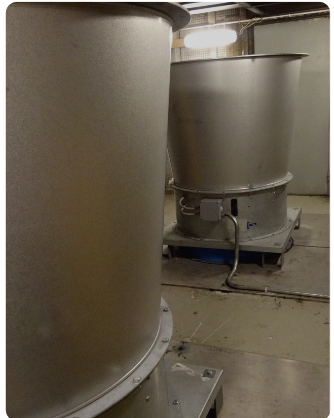
ZerAx fans supply fresh air to tunnels
