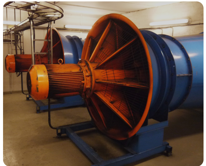
Old NOVENCO fans installed in 1980s
