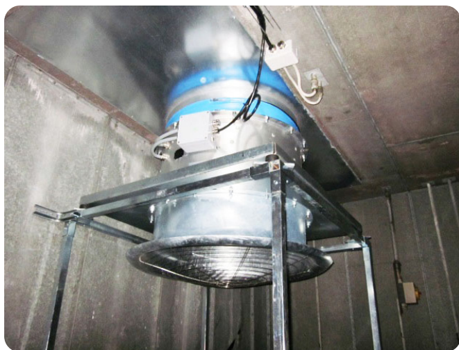
ZerAx fan installed at Carlsberg's Fredericia brewery, enhancing efficiency and reducing noise
