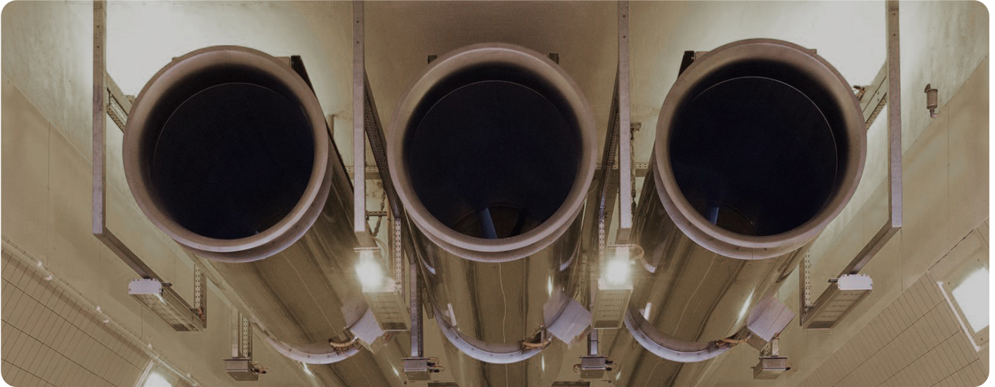
Jet fans installed at the landmark – the oldest tunnel in the Netherlands
