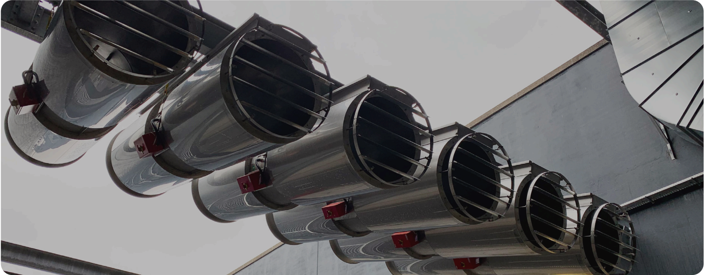
Reliable ventilation supporting safe tunnel operation
