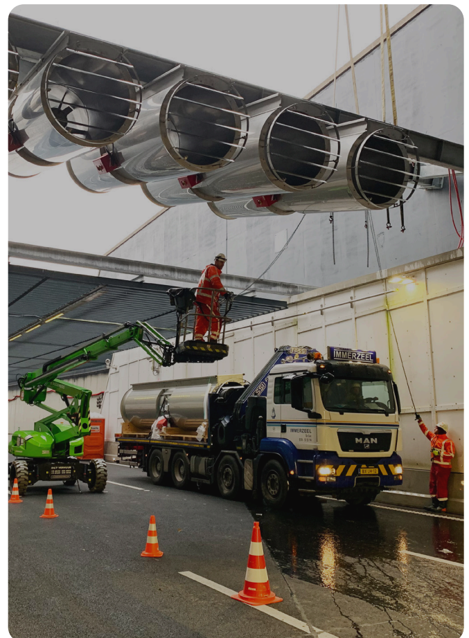
Installation of NOVENCO fans along the tunnel ceiling for ventilation and smoke control
