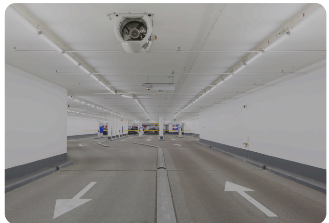
NovAx AUT-400 jet fan installed at the car park entrance
