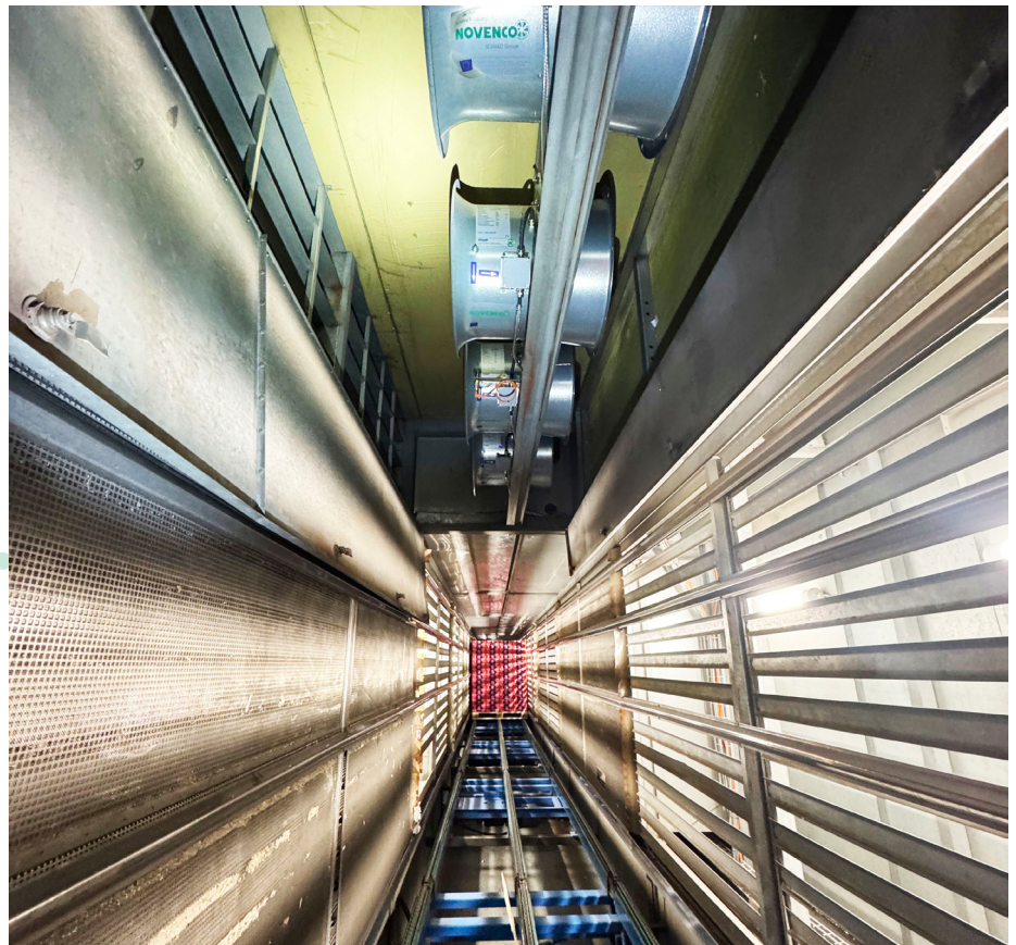
120 ZerAx® fans powering Industry 4.0 efficiency at Zott dairy
