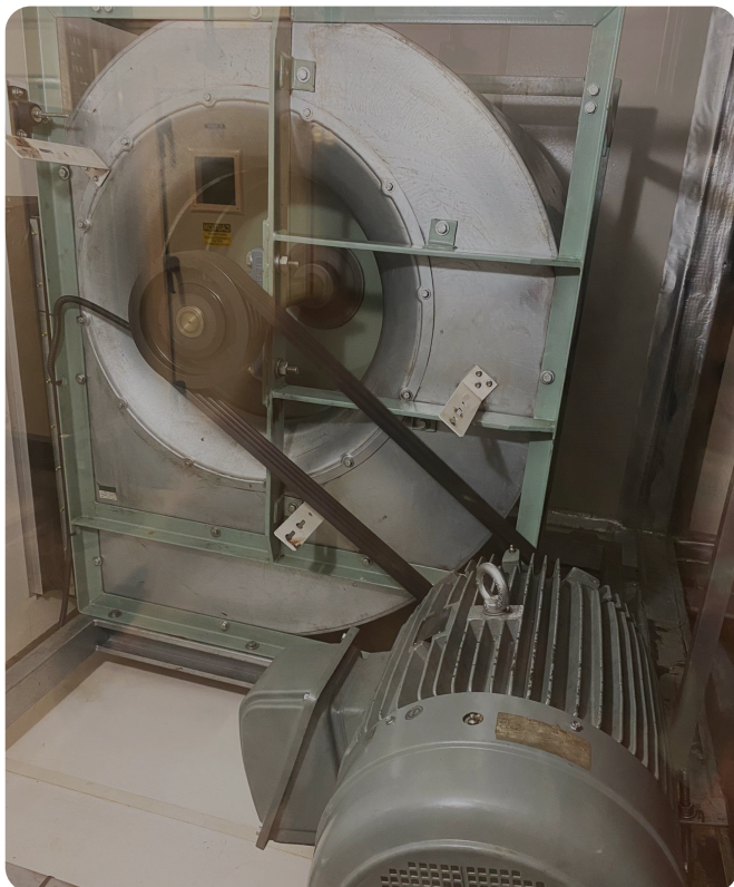
Before retrofit: the original fan installation in operation
