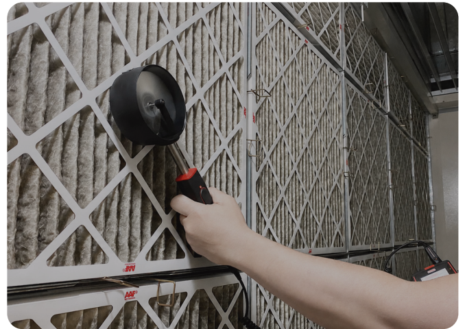
Measurement in progress on an air handling unit.
