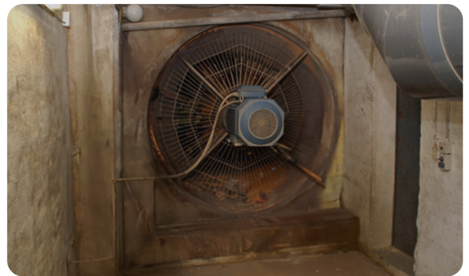
Old fan installed in the 1950s - 1960s
