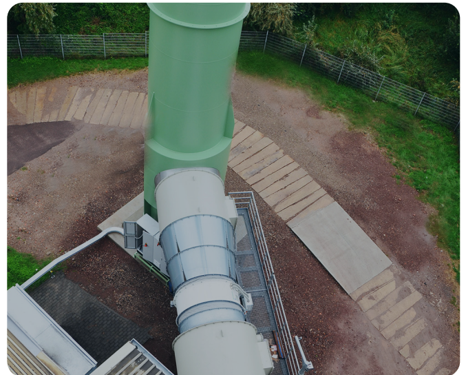
View on the new ventilation system from above
