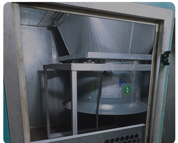
ZerAx axial fan in action, replacing the outdated fan
