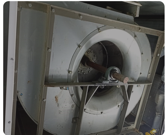
Outdated centrifugal fan before the upgrade
