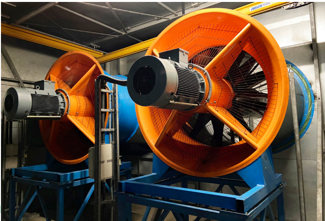
The old fans from chamber 1 The diffusers were reused
