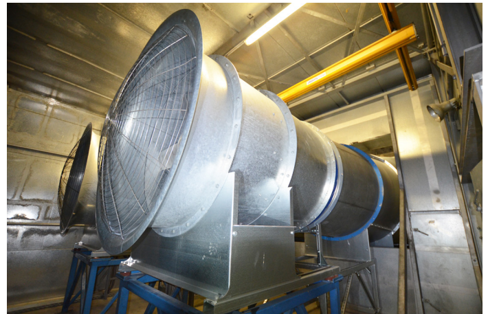
The newly mounted ZerAx® axial fans optimised for the existing plant to utilise the dynamic pressure
