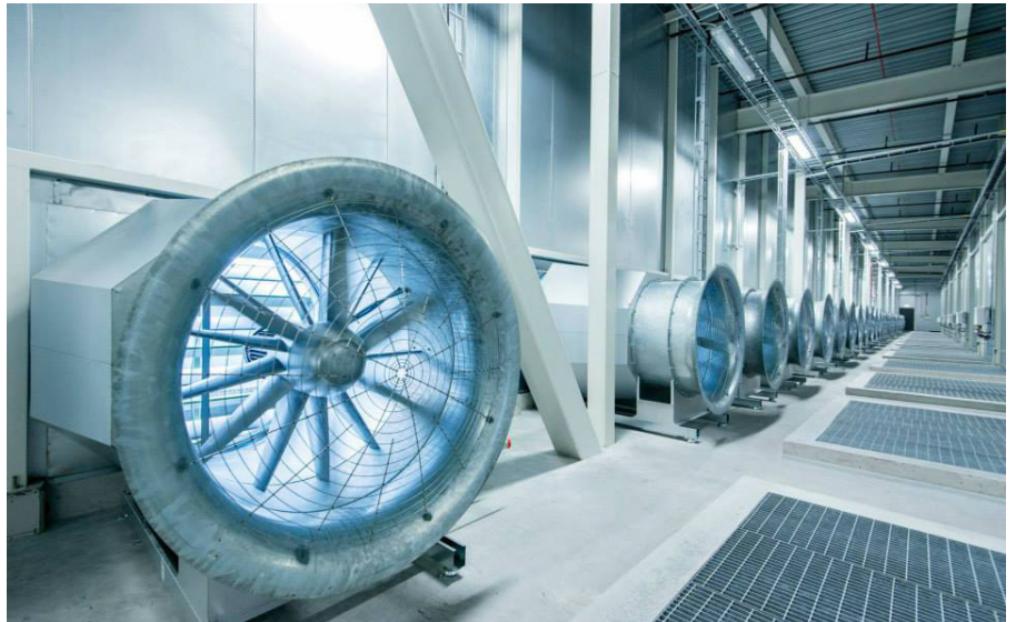
ZerAx® fans installed and ready to be used
