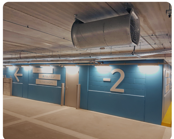
Keeping the car park safe with NOVENCO jet fan technology
