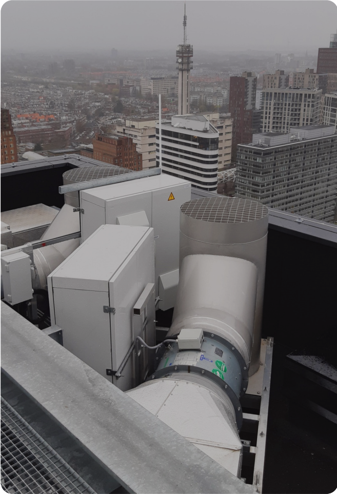
System installed on the rooftop
