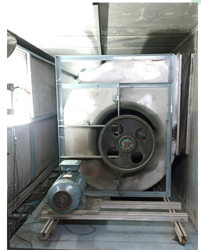
Centrifugal fan from the 1990s characterised by relatively poor energy efficiency due to outdated technology.
