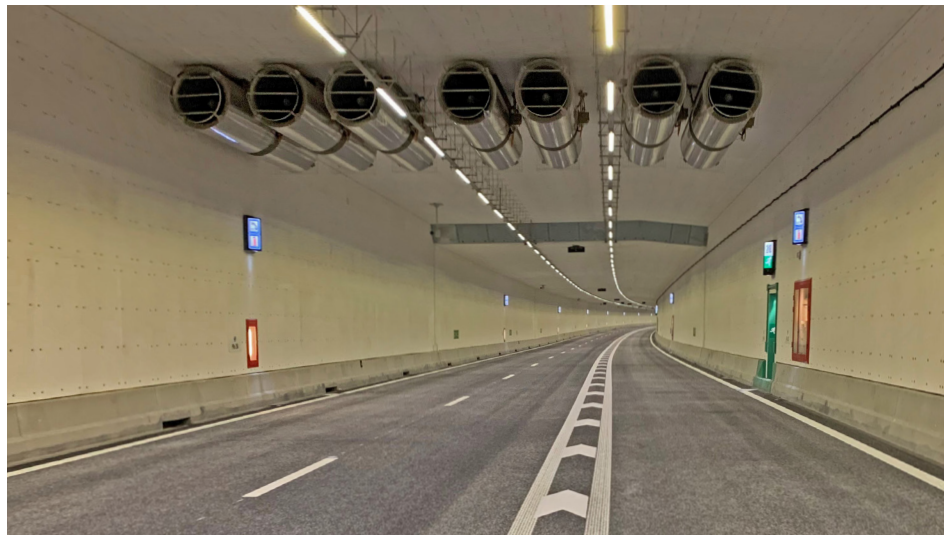
NOVENCO reversible tunnel jet fans in the Gaasperdammertunnel
