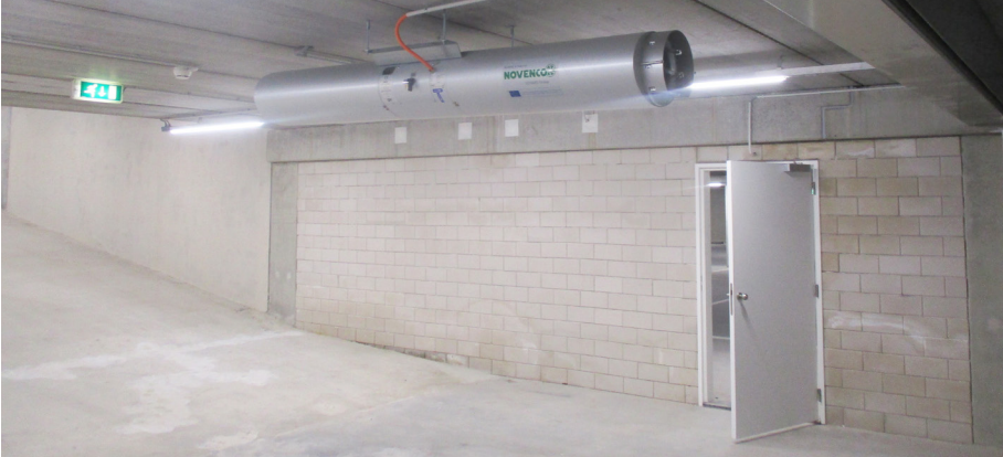
Jet fan AUO 290 in underground car park
