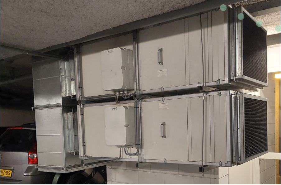
The old ventilation system with centrifugal fans
