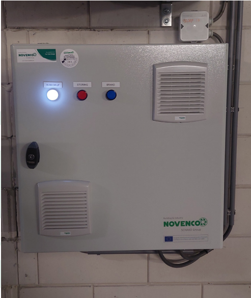
New control panel with frequency inverters and PLC
