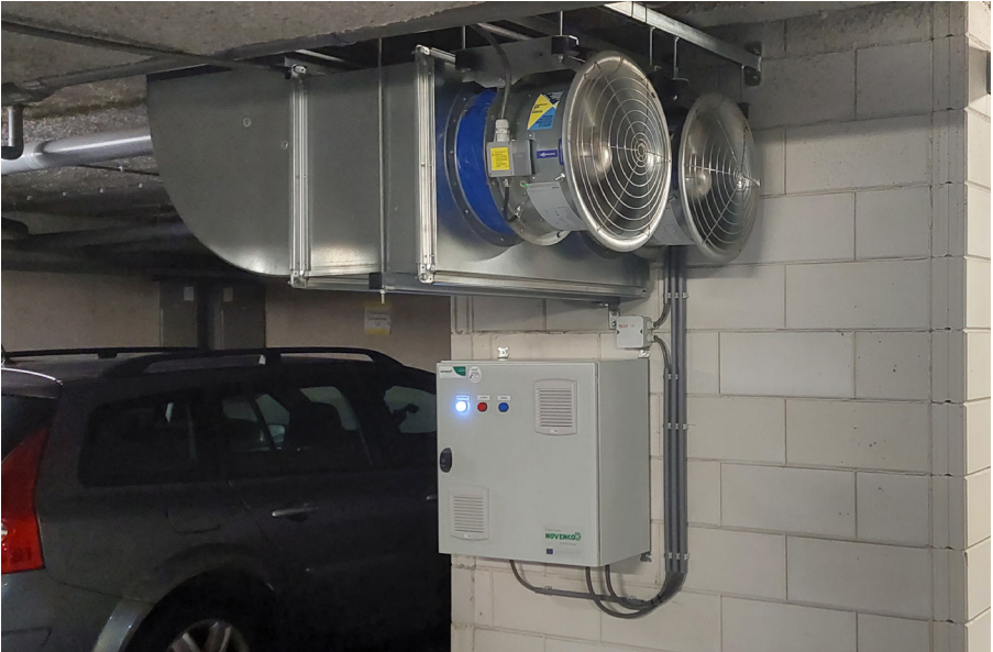
The new ventilation system with space-saving variable speed NOVENCO ZerAx fans
