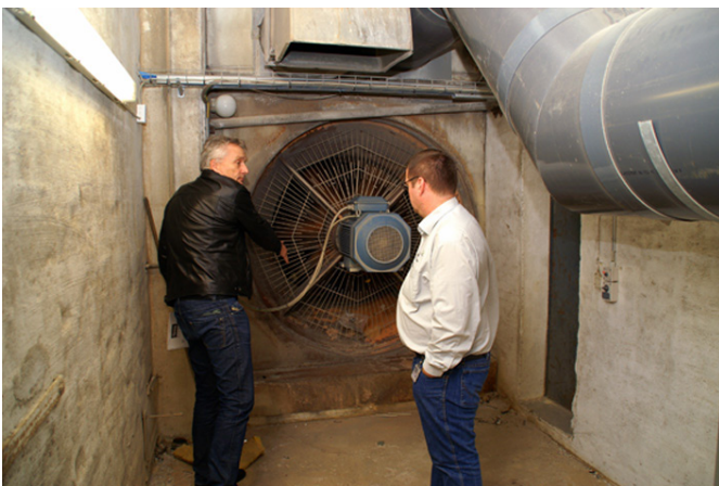
Old fans installed in the 1950s and 1960s
