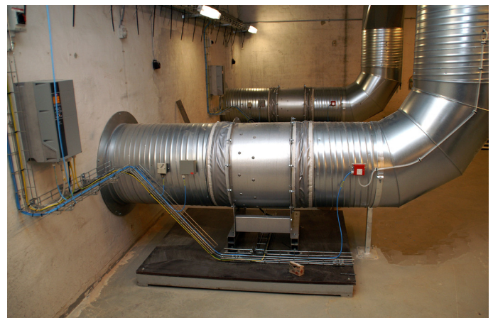
ZerAx fans installed at the Odense University Hospital
