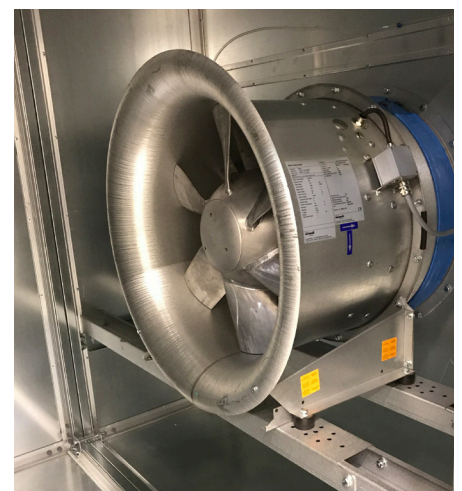
ZerAx® AZL built into AHU
