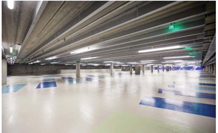
24 AU0 Jet Fans keep the Kvaesthus car park air clean from CO/NOx and CH and take care of smoke exhaust after fire
